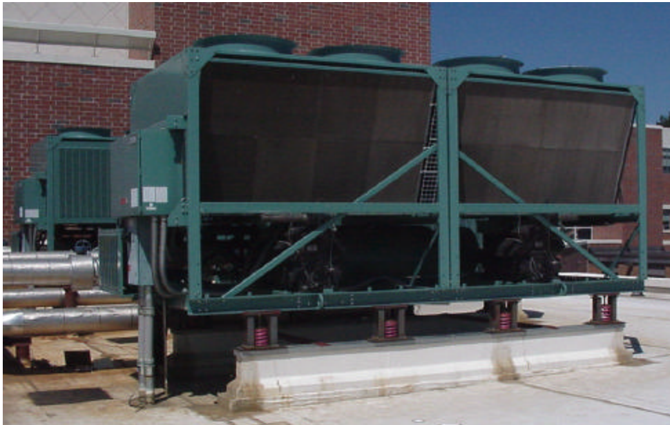
Figure 1. A reciprocating air conditioning compressor and chiller mounted on a flexible roof, Note the straight conduit on the left which bypasses the isolators and directly transmits vibration into the roof
